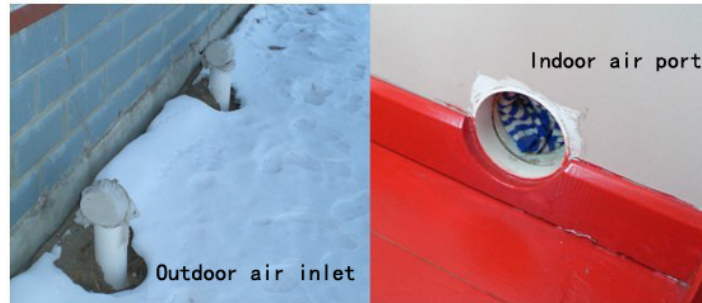
FIGURE 3: Typical Residential into Fresh Air Facilities Plugging Phenomenon.
